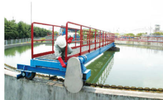
Waste Water Treatment Plant
